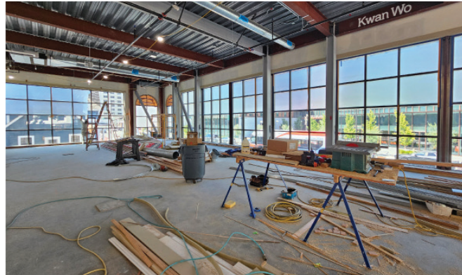
The permanent exhibition floor of the Carriage House under construction. Photo by Carmen Blair.
