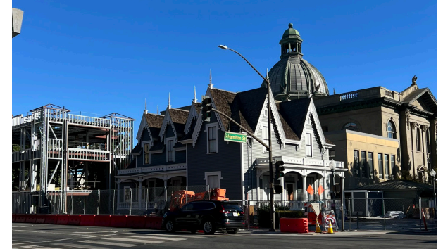
Under construction: The 15,000-square-foot Taube Family Carriage House and Automobile Gallery. Under renovation: Lathrop House.
