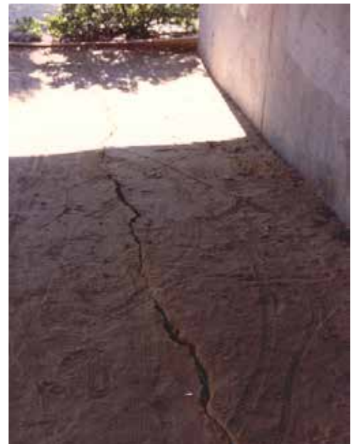
Crack under the bridge.
