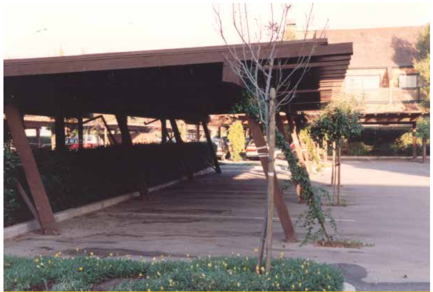
Leaning carport at the Pelican Cove condominium.
