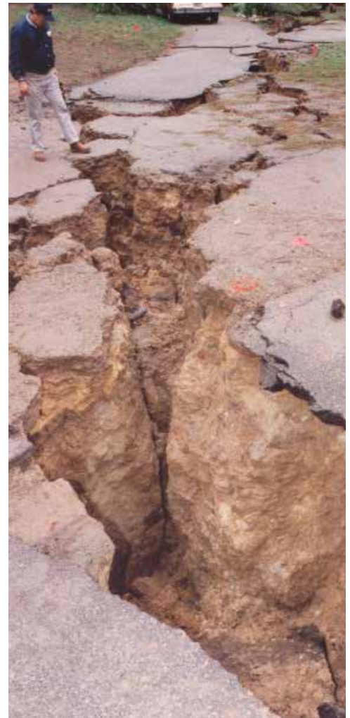
Six to ten-foot deep fissure near Summit Road.
