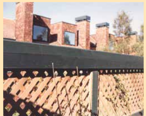
Split beam on patio at Jeff and Marsi's condominium in Redwood Shores.
