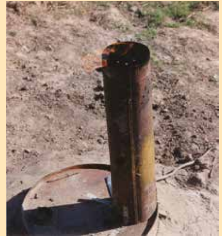
Gas leak in Pescadero.
