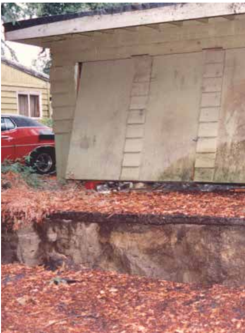
The ground lowered three feet in some areas. The fissure continued down the Country Road.
