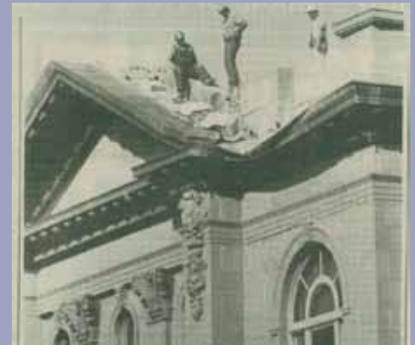
John Morgan (r) on the courthouse roof after the 1989 earthquake. Courtesy of the San Mateo County Times .
