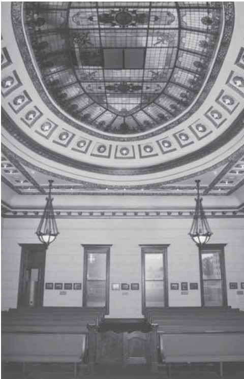
For decades, Courtroom A had an air-conditioning unit in the middle of its stained glass ceiling.
